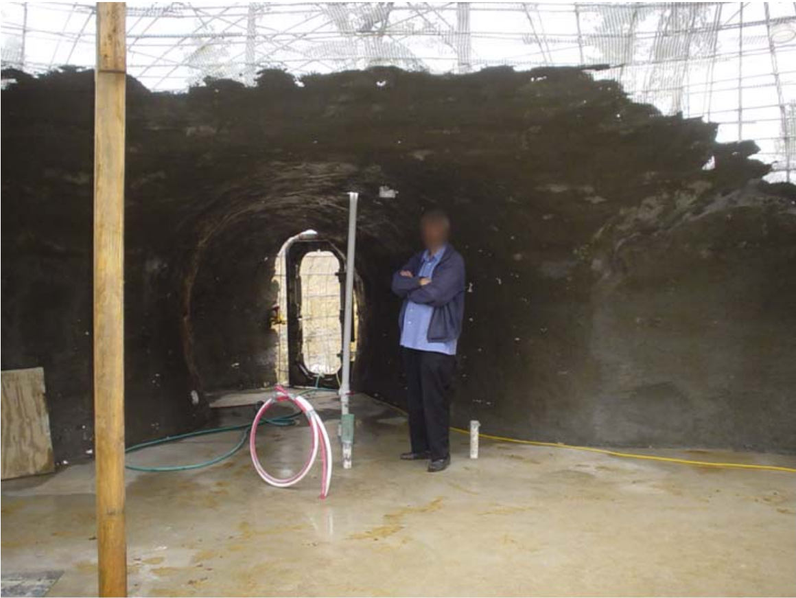
The shell being plastered up. The marine door is seen at the end of the entrance tunnel
